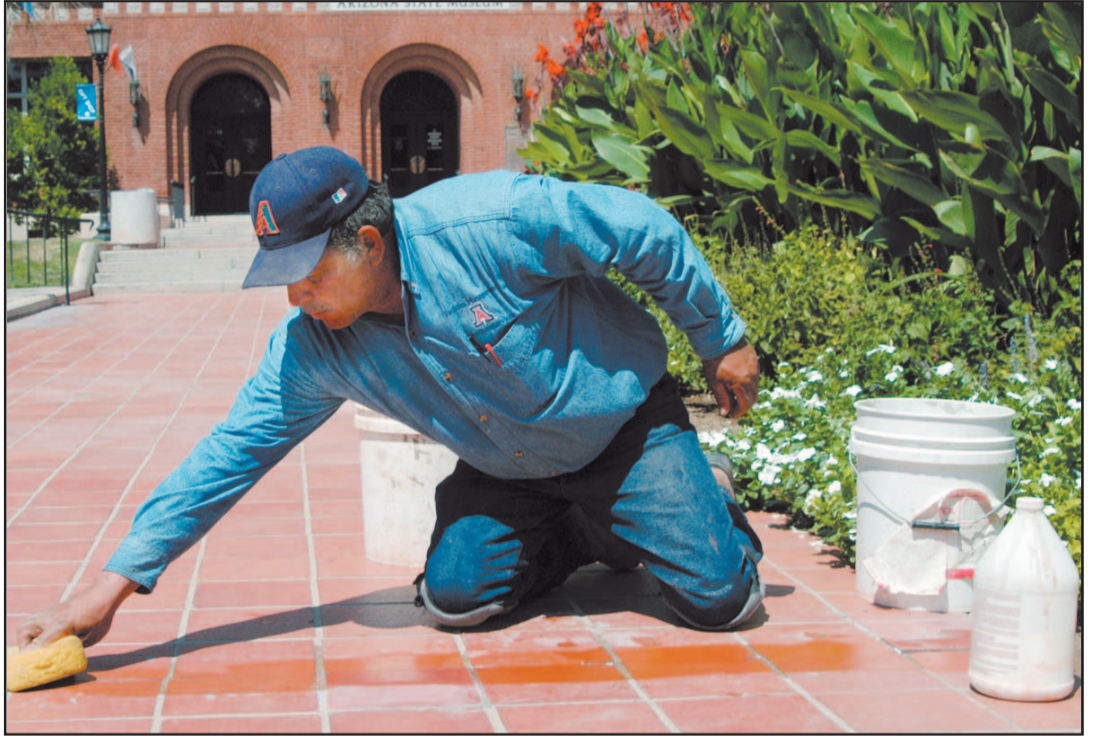
UA maintenance worker Chuy Gutierrez works under the early afternoon sun restoring the pathway in front of the Arizona State Museum yesterday. The university's brick and tile architectural details require constant care. DEREKH FROUDE/Arizona Daily Wildcat
