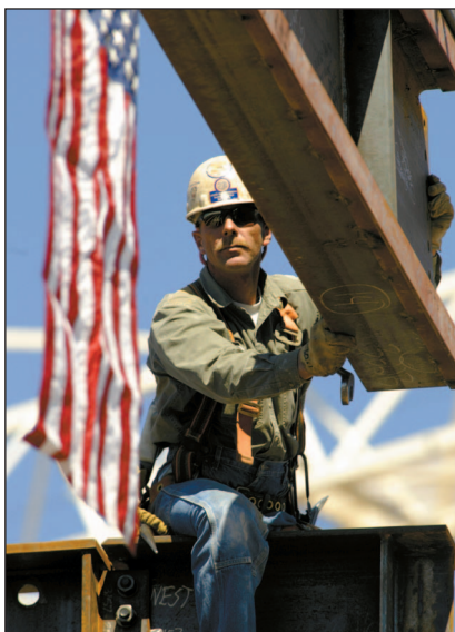
KEVIN B. KLAUS/Arizona Daily Wildcat A final beam is added to the Thomas W. Keating building yesterday. The building is expected to be completed in early 2006.
